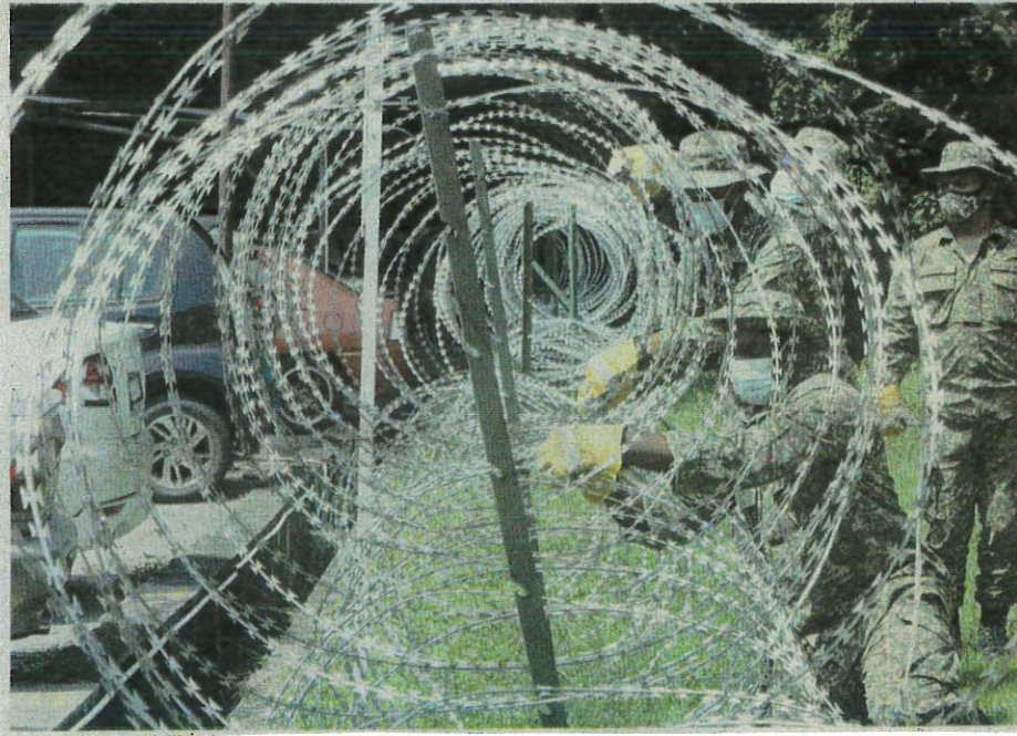
The Penang Military Reserve Force installing barbed wires at Desa Bistari Flats in Batu Uban, Georgetown yesterday after an enhanced movement control order was enforced in the area. - MASRY CHE ANI/THESUN
